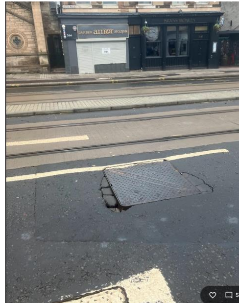
Photo taken NOV 23, barely six months after "start of revenue service": worn out lines, previous repair attempts, against A-listed building in the background; not the high-quality environment we were promised (damage still there and getting worse)
