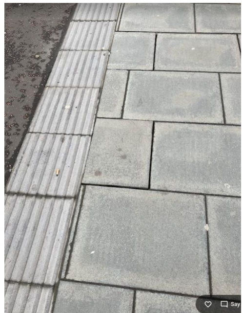
Another hidden defect : a rocking slab near a floating bus stop (where one expects extra high quality); possibly caused by Decaux's post-hoc installation of a custom-made bus shelter. Who is responsible? Who pays? When will it get fixed?
