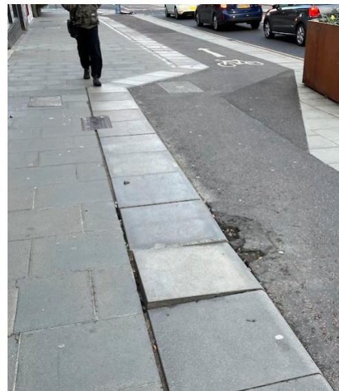
Very narrow pavement in area of high footfall; post hoc widened for cyclists following international press coverage (is remaining space for the planter really necessary?); rocking slab is a hazard for pedestrians; potholes near lip increase risks for cyclists
