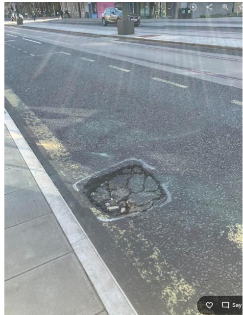
Sinkhole near busy bus stop (with decaying lines), no iron work nearby; if caused by collapsed pipe below, how many of these hidden defects will emerge before the end of the defects period?
