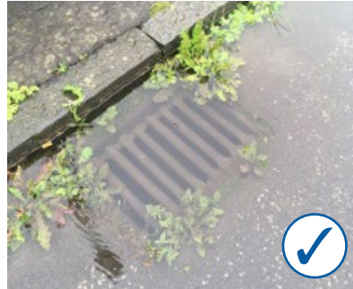
Gully clear but flooding during 'normal' rainfall
