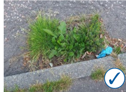
Gully blocked with vegetation
