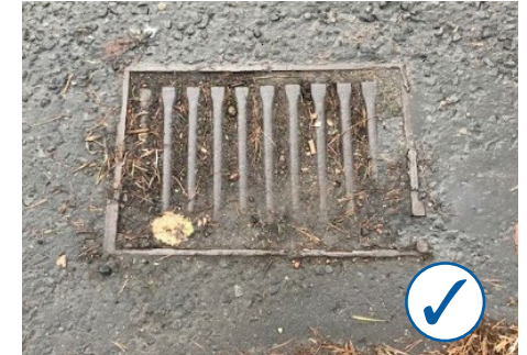
Gully full of silt
