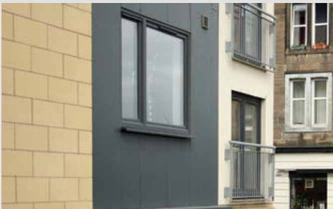
Too many materials The cladding, blockwork and render and their detailing used at this development would not now meet the Council's expectations for appropriate quality.
