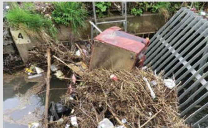
locked up culvert
