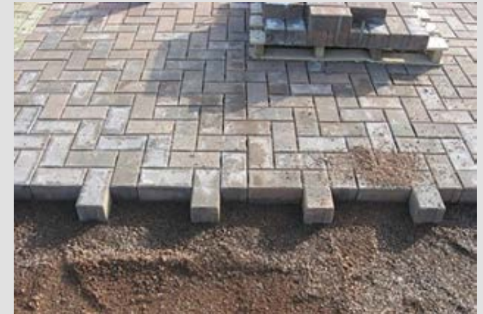
Shared surfaces outwith conservation areas Shared surfaces outwith conservation areas need to be kept very simple. If block paving is used, there should be no more than two tones and these should be grey.
