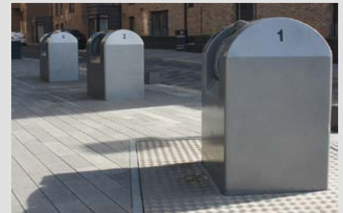
Underground bins for residual waste allow large volumes to be held with minimal impact on the street scene. It is important that the Council's Waste and Cleansing Service are involved early, as their requirements may impact on the design.
