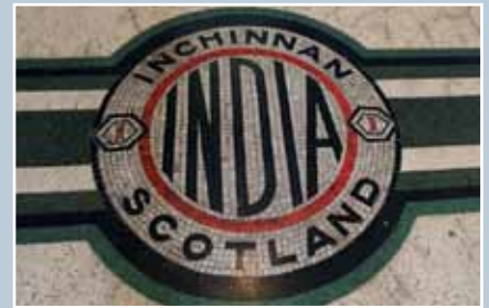
Former India of Inchinnan Tyre Factory of 1929–30, Renfrewshire. The mosaic floor was conserved and the cracks sealed as part of the rescue of this building at risk.
