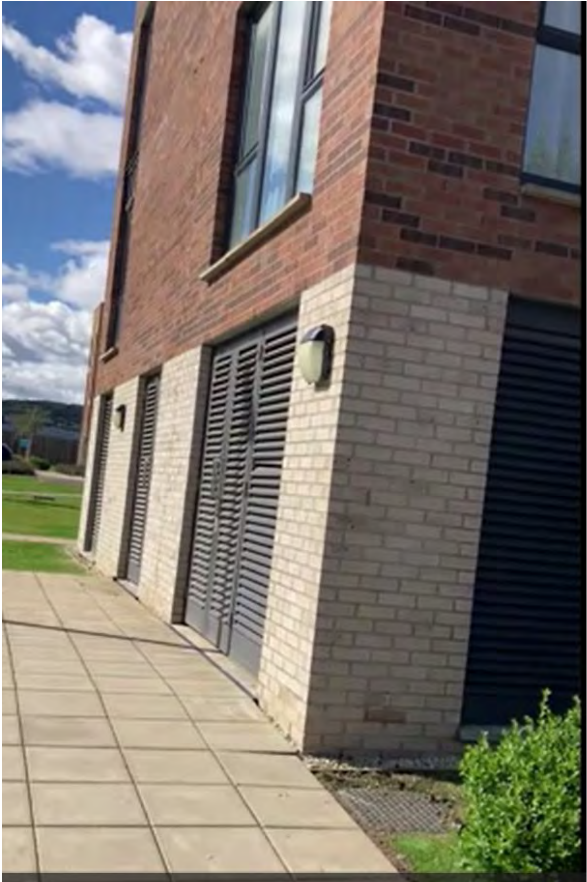
Louvre doors to refuse store, plant room & bike store located below windows of Flat 5 above.
