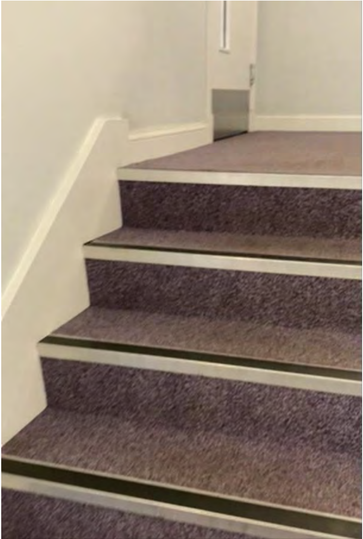
Carpeted stair, first floor landing and sealed fire door leading to inner hallway.
