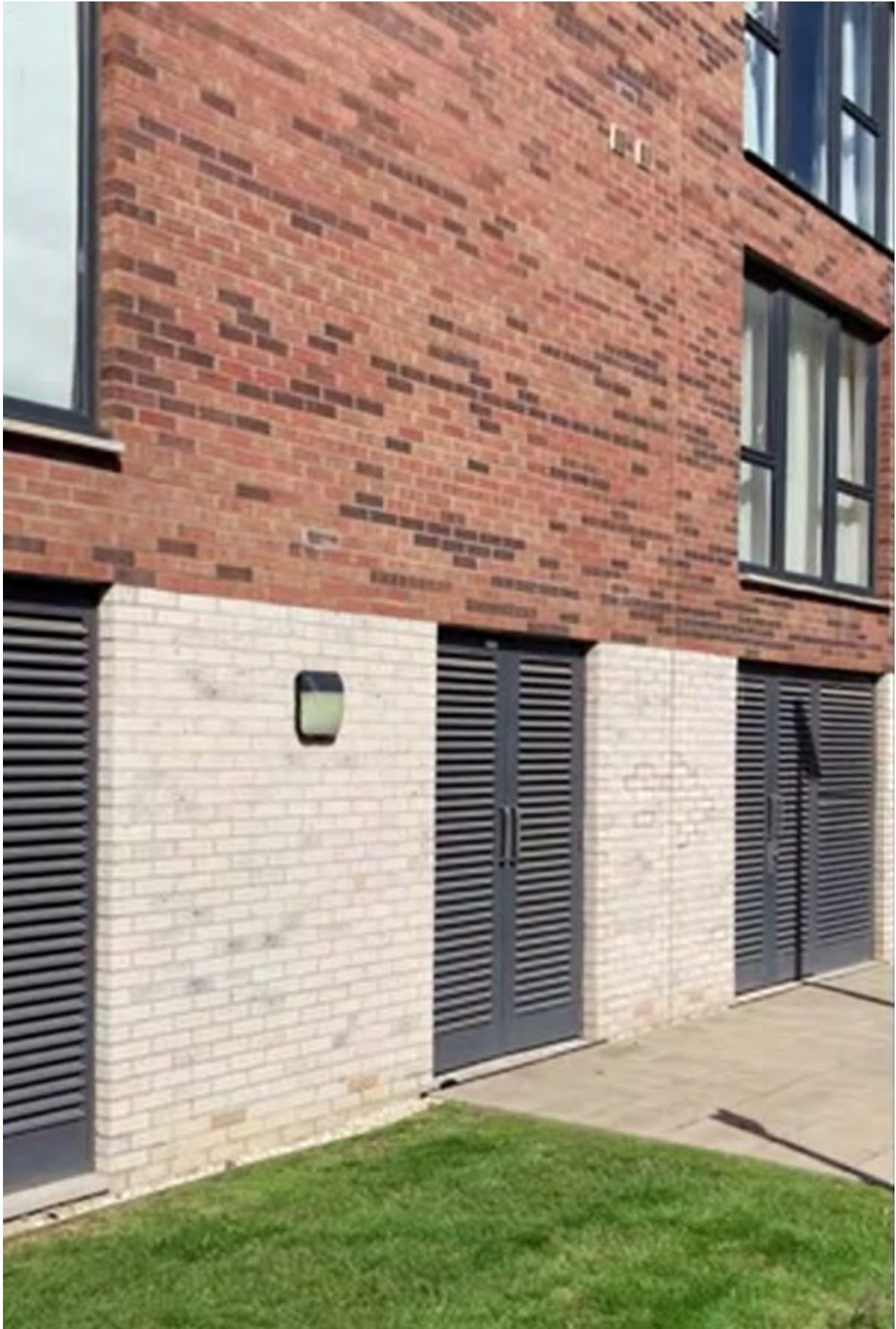
Reverse image of bike store, plant room & refuse store with Flat 5 windows above.
